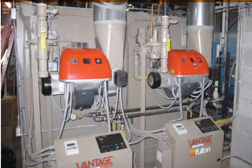
The Laughlin Memorial Hospital in Greeneville, Tennessee replaced their existing steam boilers with four Fulton Vantage 4.0 MM Btu/hr boilers and a custom ModSync controller. Photo courtesy Fulton Boiler Works.
