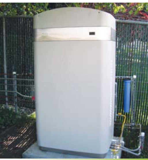
Installation of a ClearEdge 5 kW unit serves an office complex in Florida, and also generates 700-800 gallons of hot water per day.
