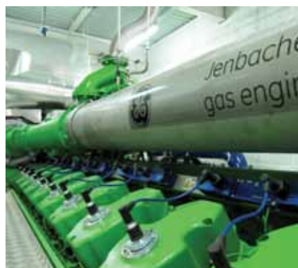
This 620 Jenbacher engine-generator set is installed in a Coca-Cola plant in Romania.
