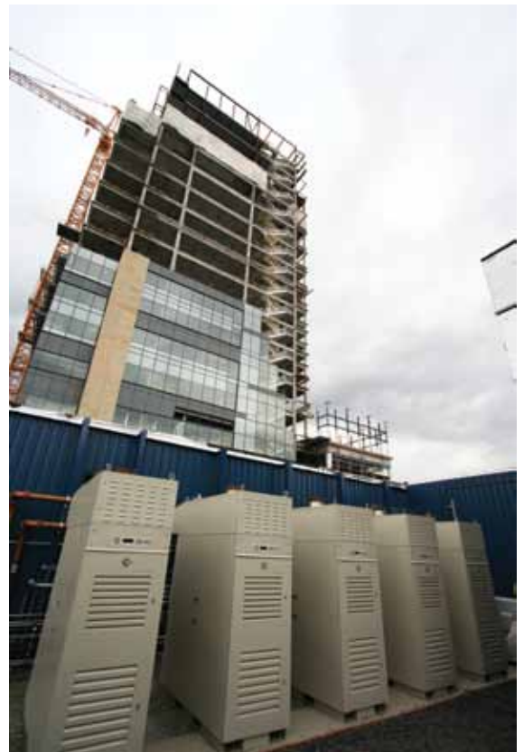
The Oregon Health Science Center is equipped with five Capstone microturbines, supplying both electric power and hot water.
