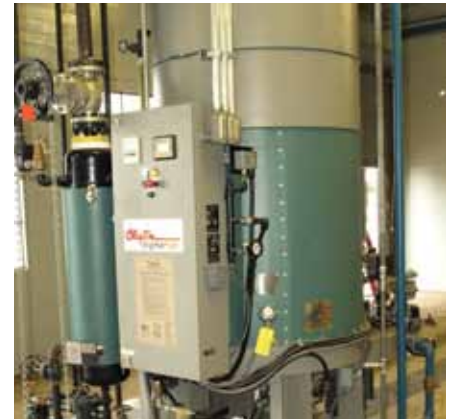
Today's packaged boilers, such as this Clayton unit, are very compact, allowing expansion of mechanical plant capacity in the same floor space.
