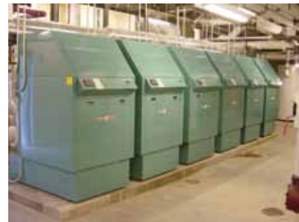
By installing multiple condensing boilers such as these Cleaver Brooks ClearFire units, plant efficiency can be maintained in the “sweet spot” through the year, while also allowing redundant capacity for simplified unit maintenance.
