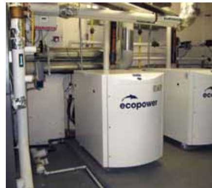
Two Marathon Engines cogeneration units are installed in a multi-family residential building in the City of New York.
