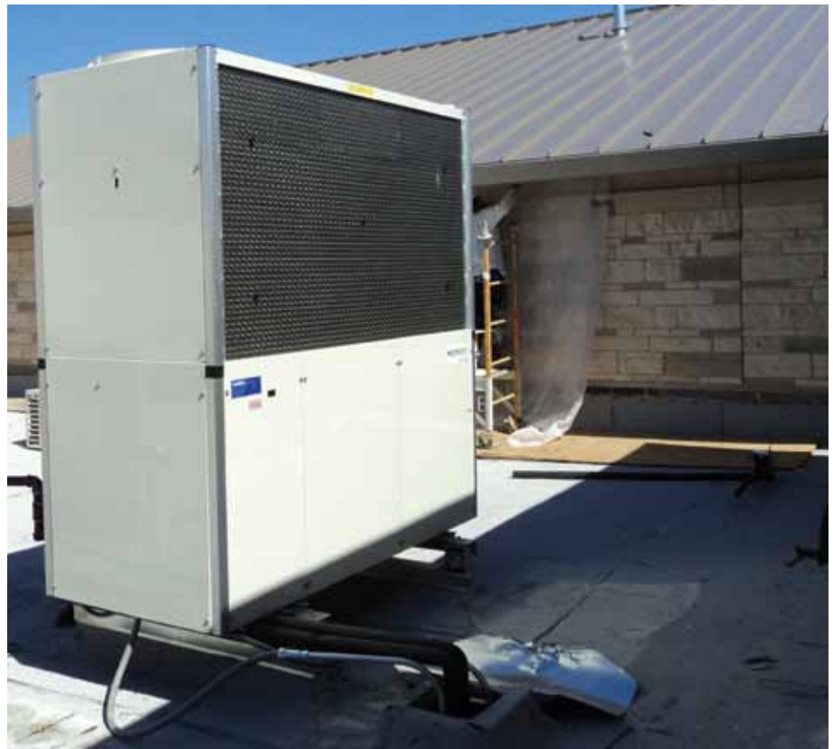
The 15-ton heat pump installed at Plano (TX) Fire Station No. 13 offers the opportunity to test the operating costs of gas vs. electric cooling. Energy use and cost at the station will be compared with that of another "twin" station using electric cooling technology.
