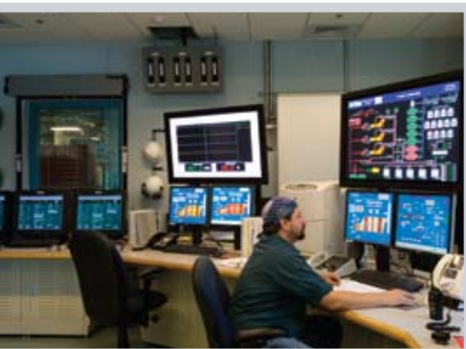
Control area for three gas turbine generator sets in a combined heat and power application at a university in Connecticut. Photo courtesy Solar Turbines.
