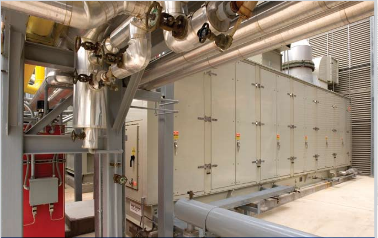
A recuperated gas turbine providing heating, cooling, and power at hospital in Texas. Photo courtesy Solar Turbines.
