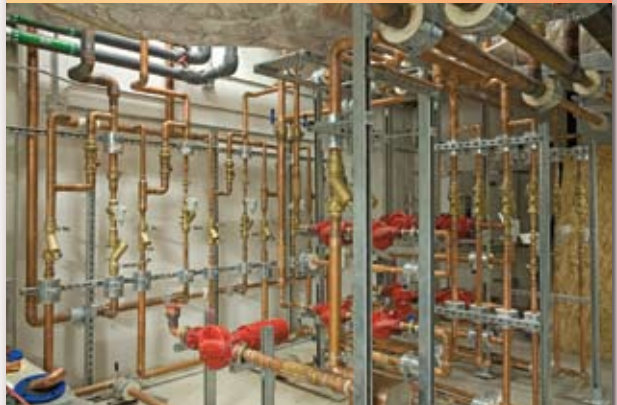
In most radiant floor applications, each floor has multiple zones, allowing flexible control of heat levels as building use changes. Photos courtesy Uponor.
