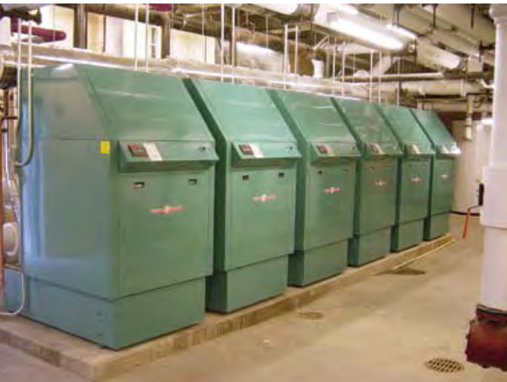
Often replacing an oil-fired boiler is an opportunity to go to a modular gas-fired boiler system. Here six 1,800 MMBTU gas fired ClearFire-C boilers replace an older oil-fired unit in an educational building. Photo courtesy Cleaver-Brooks.
