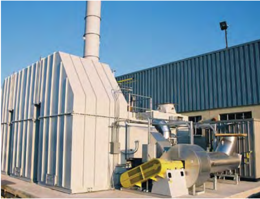
A 22,000 scfm rotary concentrator with a three-chamber regenerative thermal oxidizer is designed for high destruction efficiency. Photo courtesy Catalytic Combustion Corporation.
