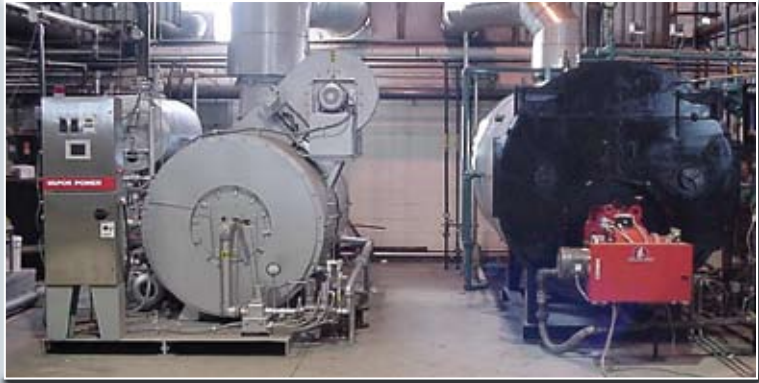
Coil tube boilers fit in well with existing plant units. Here a 450 bhp Vapor Power Circulatic® horizontal coil tube boiler stands alongside a 250 bhp firetube boiler. Note also the similar footprint for the larger capacity coil tube boiler. Photo courtesy Vapor Power.
