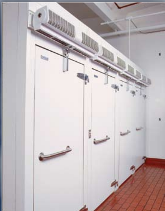
➤ Another ideal energy saving installation is in front of refrigerated and freezer areas. Photo courtesy Mars Air Systems.
