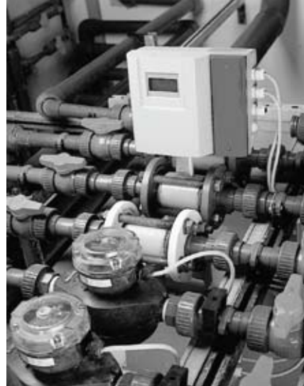
Digital flow meters installed at a potable water bottling plant. For this type of product metering, both accuracy and repeatability are important. Photo courtesy Badger Meter Corp.
