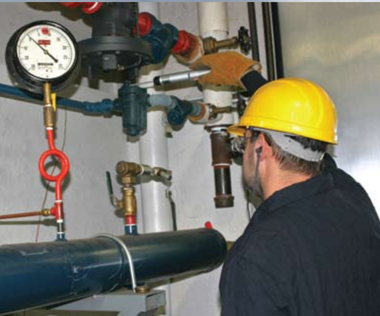
The technician is using an ultrasonic method to test an Armstrong cast iron inverted bucket steam trap. Photo courtesy Armstrong International
