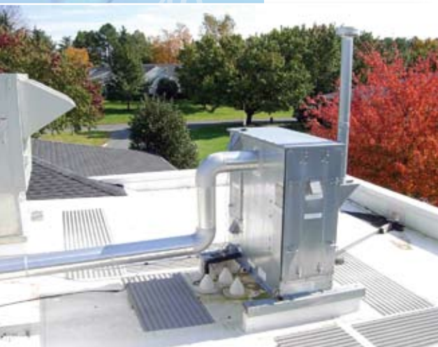
This packaged humidifier is mounted outdoors, with the output sent to an Armstrong HumidiPack unit for dispersion in an air handler. Photo courtesy Armstrong International
